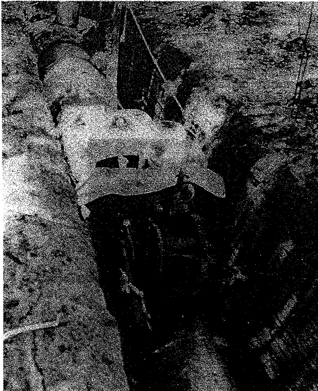
Fig. 1.2.2a — Two-stage construction by machine. Construction of 30 in. (760 mm) diameter pipe showing the machine that places the top half of the concrete pipe.
