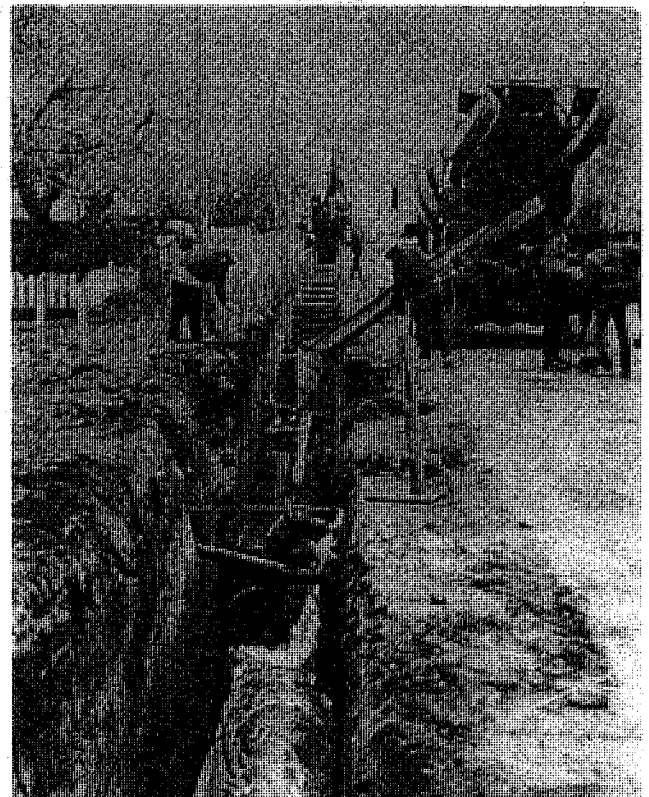
Fig. 1.2.1.1e — Single-stage construction using metal forms. A 42 in. (1065 mm) machine installing storm drain pipe. Metal forms are lined up at the side of the trench before manually lowering into machine. As pipe is formed the outside top is covered with polyethylene to retain moisture and ensure proper curing.
