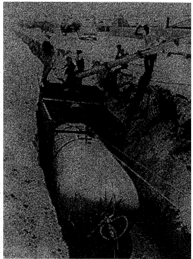
Fig. 1.2.1.2c — Single stage construction using inflatable form. Machine with inflated inner form being pulled down the trench with concrete being fed into the hoppers. As the machine moves it pulls up the form and guides it on rollers through the trench as the concrete is moved around the form with tampers and vibrators.
