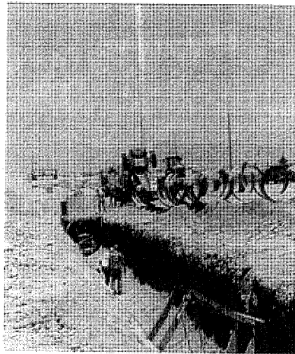
With the deadman in position, the pour continues as forms await their use. Note laser on tripod to ensure grade and direction.
