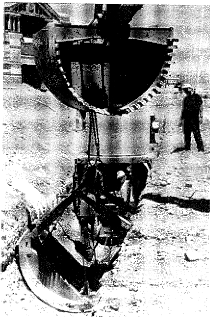
Excavator prepares to lift and move deadman farther back in the trench to continue the day's pour.
